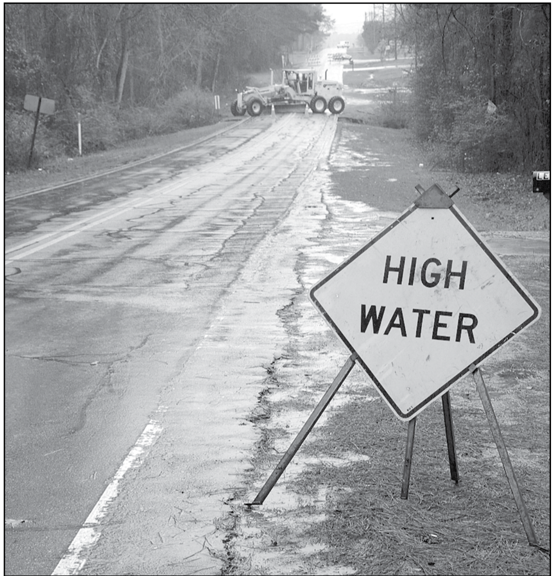
DOT blocked Lindsay Road after water eroded the roadbed.
